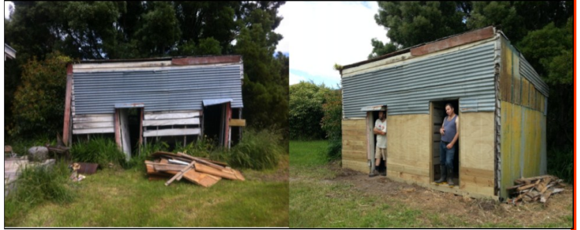
Left: Before shot Right: Kosta and Adrian after completion proving the shed's strength by leaning on the newly repositioned doorframes
