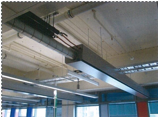
Picture 1 – Conservation House Active Chilled Beam (Photo: 12/06/2009)
