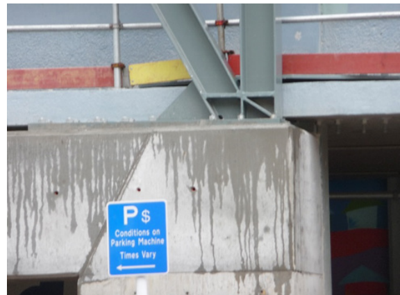
Figure 3. Connection between column and frame. The column is embedded the whole height of the RC column while a horizontal plate with many embedded bolts transfers horizontal forces into the diagonal brace.
