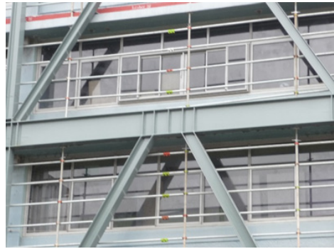
Figure 2. The short length of beam between the diagonals will be distorted when it functions as a seismic fuse.
